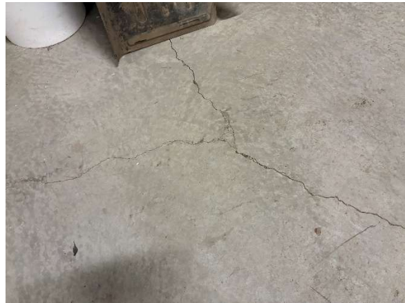
Figure 38: Main WTP Building Slab Cracking
