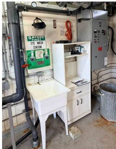
Figure 45: Bulk Water Distribution Building Utility Sink
