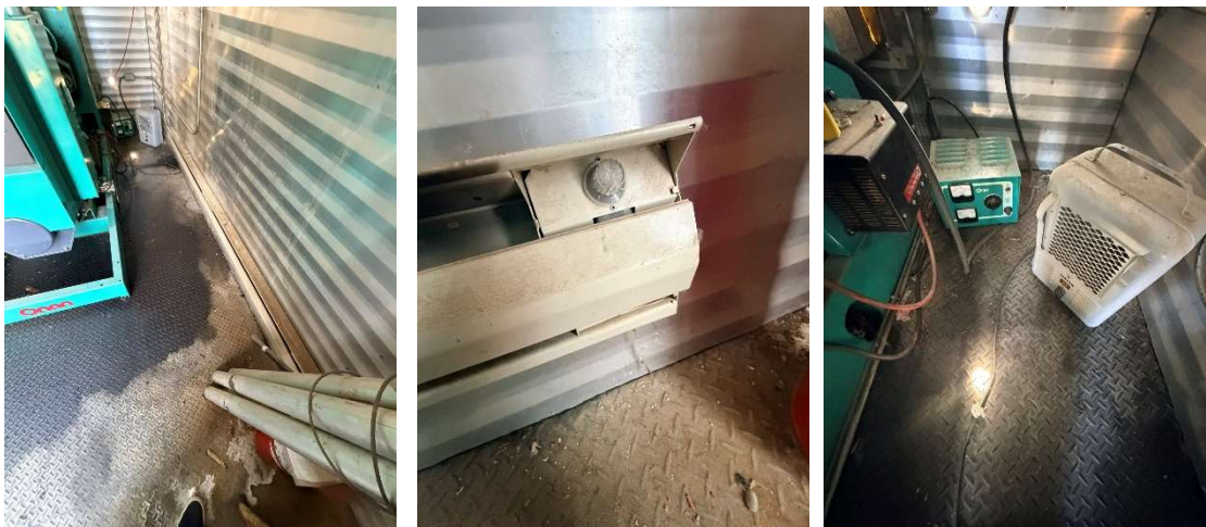
Figure 52: Baseboard Heater & Portable Heater
