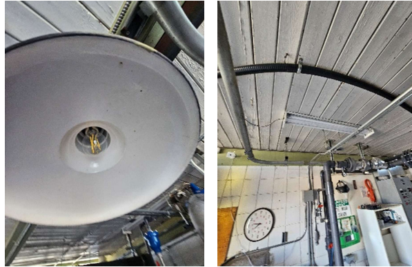
Figure 64: Fire Pump Building Existing Lighting
