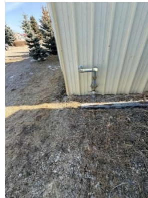
Figure 48: Gas Serving the Public Works Shop & WTP Building
