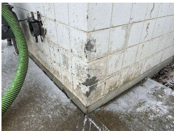
Figure 41: Bulk Water Distribution Building CMU Wall Block Abrasions
