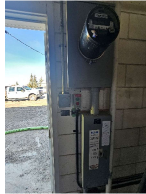
Figure 68: Utility Meter and Main Disconnect
