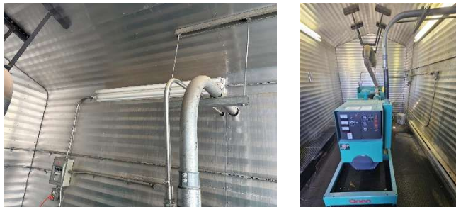
Figure 65: Generator Walk-in Enclosure Lighting
