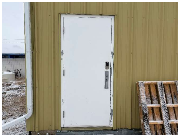
Figure 25: Main WTP Building East Door Frame Paint Flaking
