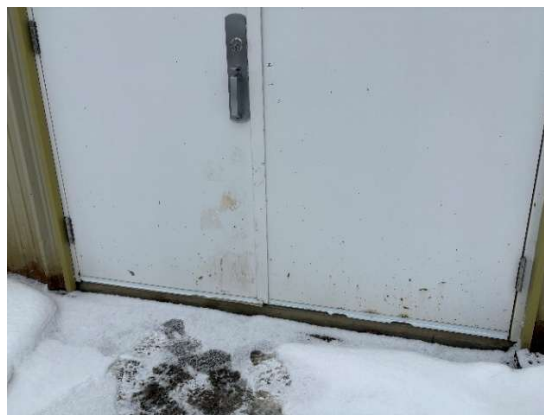
Figure 24: Main WTP Building North Man Door Deterioration
