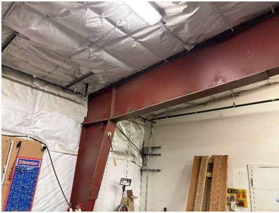
Figure 37: Main WTP Building Steel Beam/Column Weld Burns
