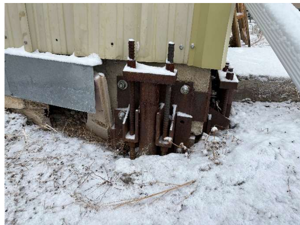
Figure 40: Main WTP Building Beam/Slab Shear Crack
