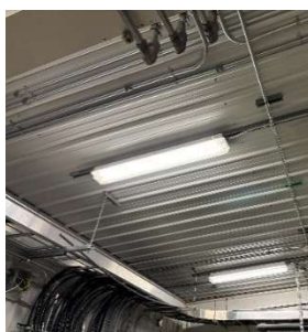
Figure 63: Water Treatment Lighting
