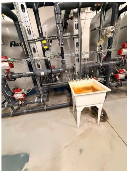
Figure 44: WTP Utility Sink
