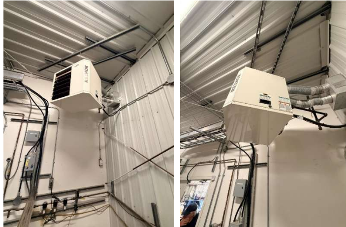
Figure 51: WTP Unit Heater (UH-3)
