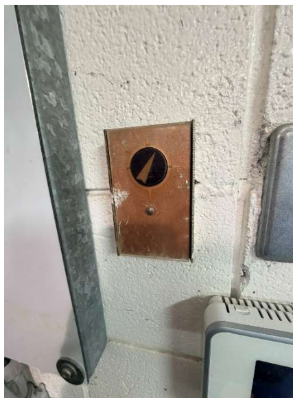
Figure 54: Unit Heater Thermostat
