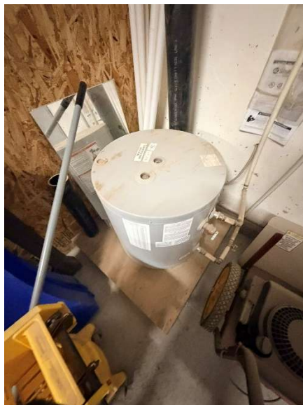
Figure 43: Public Works Shop Water Heater
