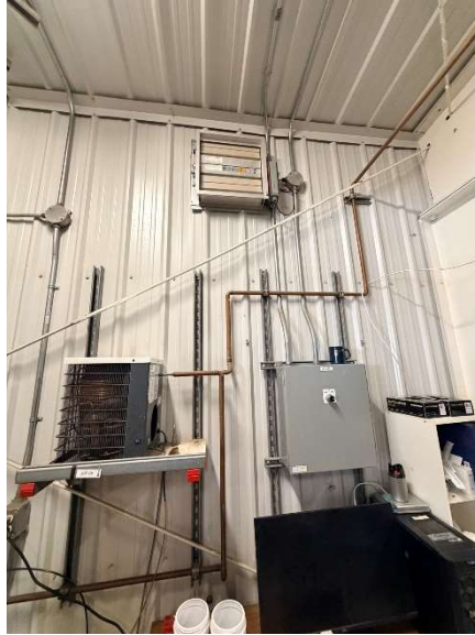
Figure 55: WTP Motorized Damper (DM-102)
