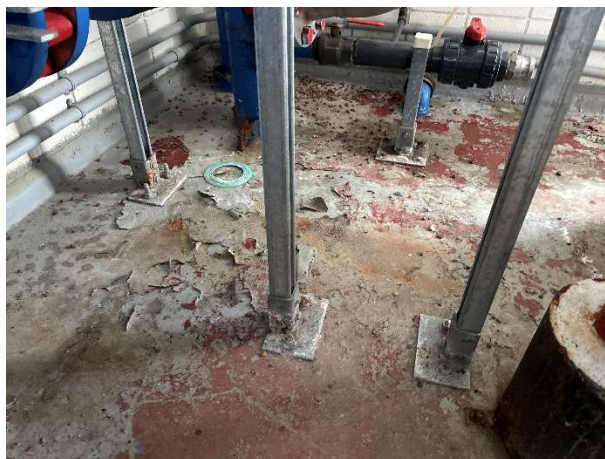
Figure 34: Bulk Water Distribution Building Slab Epoxy Finish Deterioration
