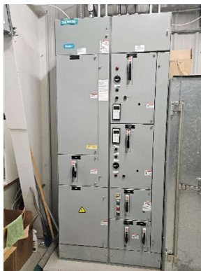
Figure 66: Motor Control Center
