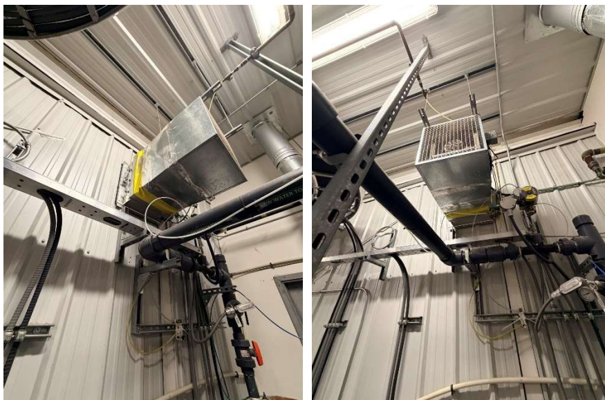
Figure 58: WTP Exhaust Fan
