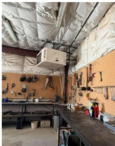
Figure 49: Typical Workshop Unit Heater
