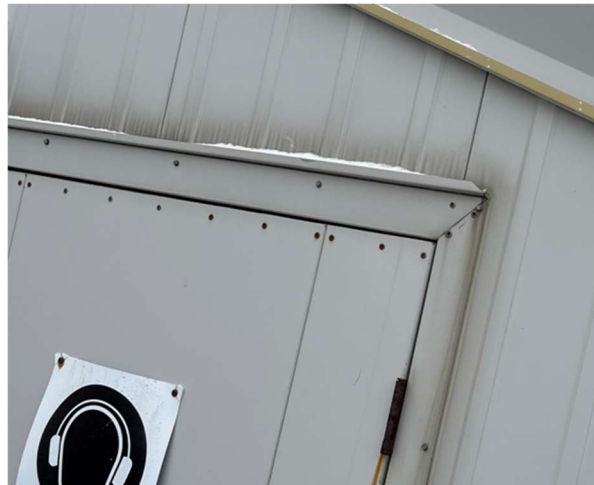
Figure 21: Generator Building Wall Cladding Stains
