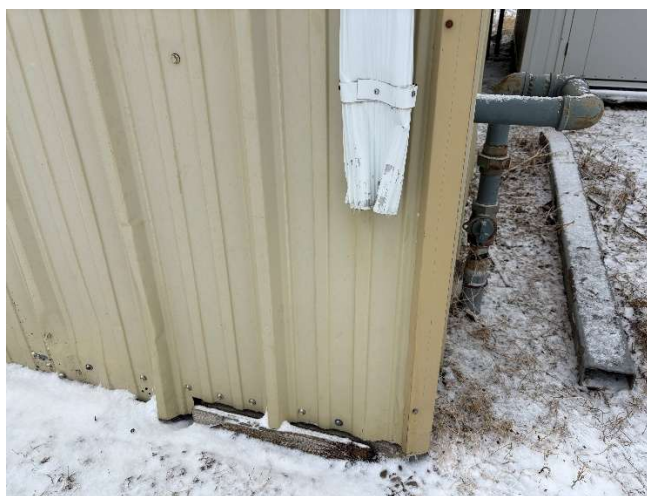
Figure 14: Main WTP Building Missing Downspout Extension
