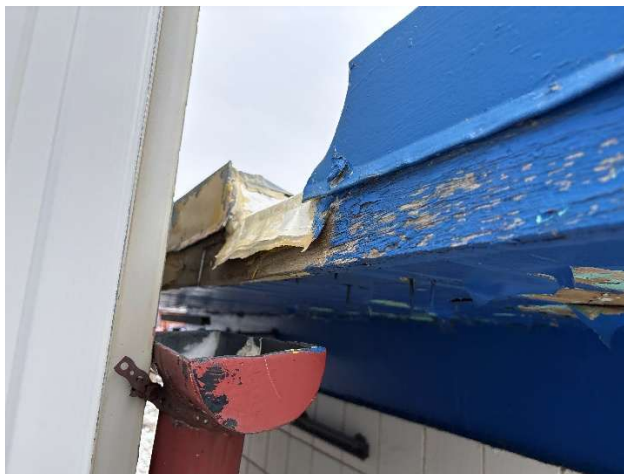
Figure 15: Bulk Water Distribution Building Roof Drainage System
