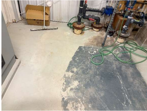
Figure 30: Main WTP Building Slab Epoxy Finish Deterioration
