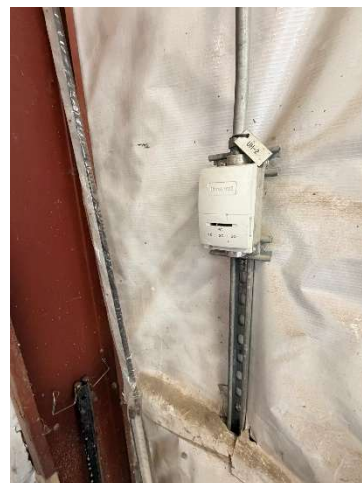
Figure 50: Typical Unit Heater Thermostat
