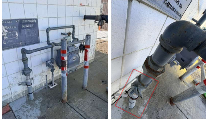
Figure 46: Bulk Water Distribution Building Gas Service
