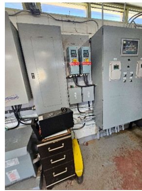
Figure 70: Main Distribution Panel and Control Panel
