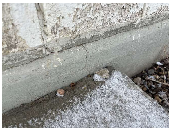
Figure 42: Bulk Water Distribution Building Foundation Cracking
