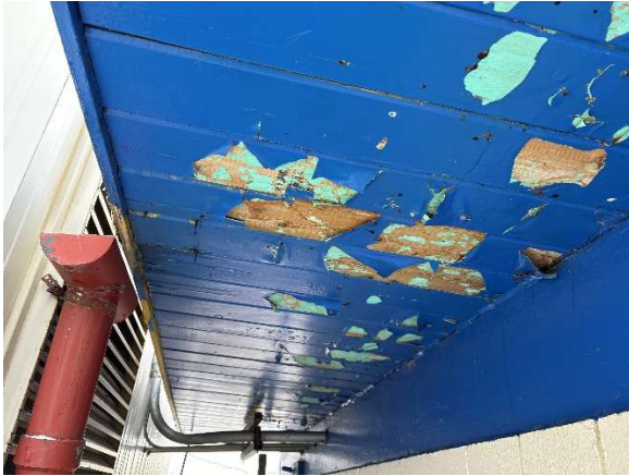
Figure 19: Bulk Water Distribution Building Wood Soffit Paint Flaking
