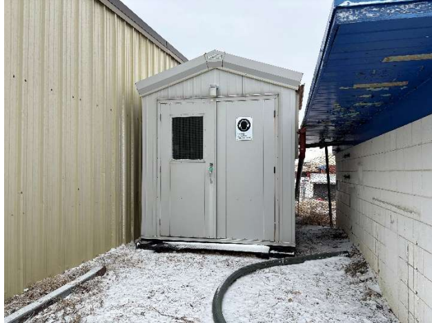
Figure 13: Generator Building Skid
