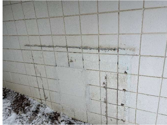
Figure 20: Bulk Water Distribution Building CMU Block Wall Scuffs
