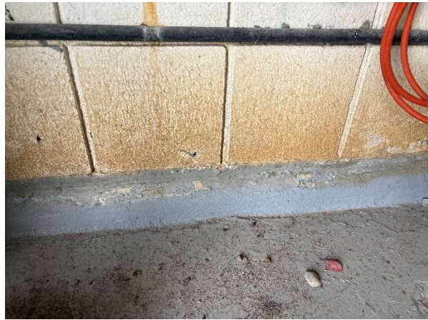
Figure 32: Bulk Water Distribution Building Worn Out Wall Paint
