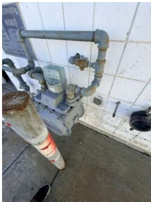
Figure 47: Gas Service Entering the Pump Station
