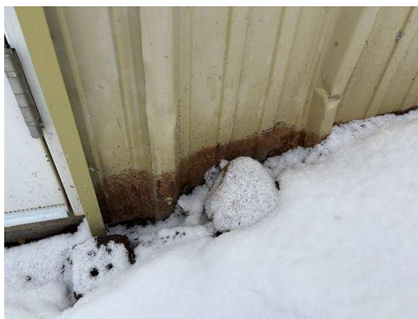
Figure 18: Main WTP Building Cladding Corrosion
