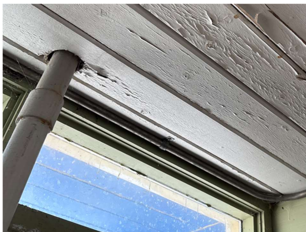
Figure 26: Bulk Water Distribution Building Window Deterioration
