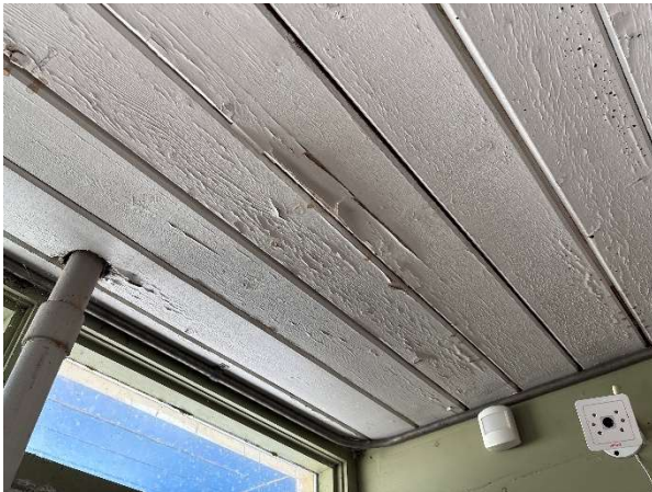
Figure 31: Bulk Water Distribution Building Ceiling Paint Flaking
