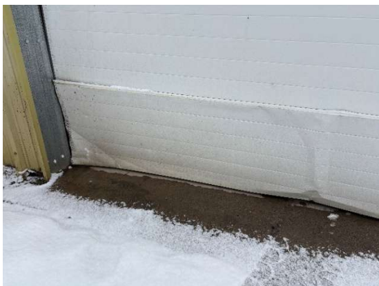
Figure 23: Main WTP Building North Garage Door Damage
