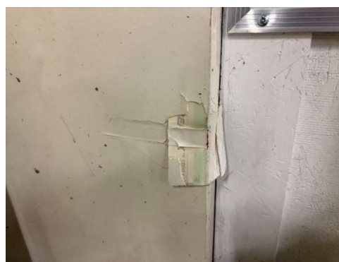
Figure 29: Main WTP Building Drywall Damage
