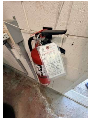
Figure 61: Typical Fire Extinguisher
