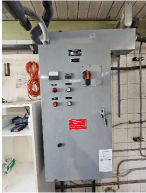
Figure 67: Fire Pump Controller
