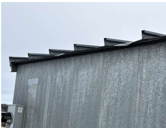
Figure 8: Roof Decking Warping
