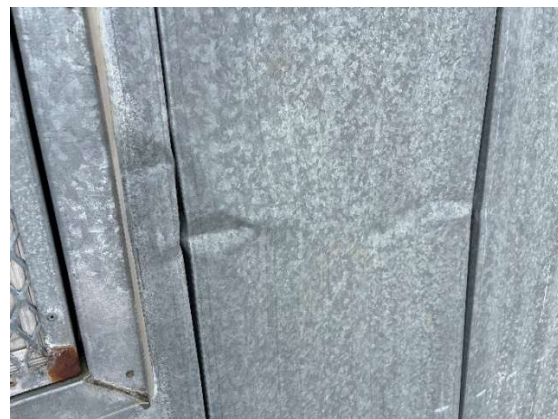
Figure 9: Wall Cladding Dents
