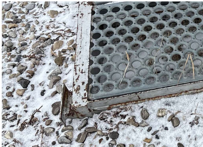
Figure 15: Steel Skid Corrosion
