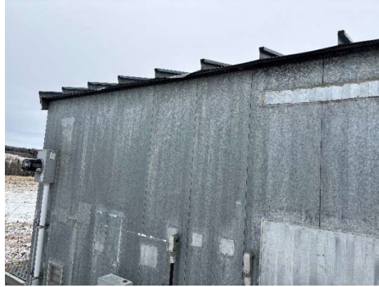
Figure 7: Missing Roof Drainage System
