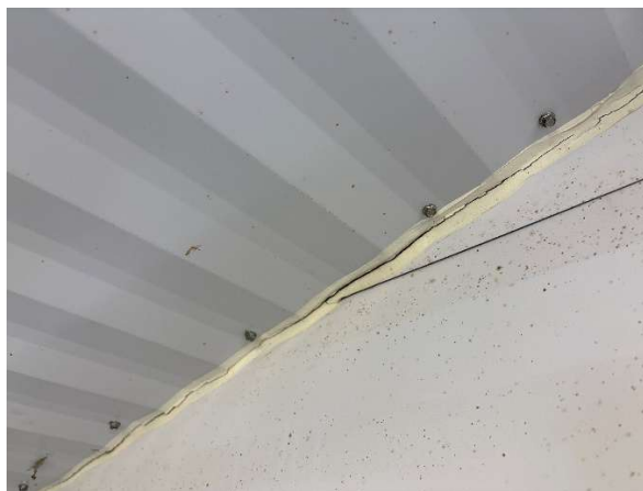
Figure 13: Cracked Joint Caulking
