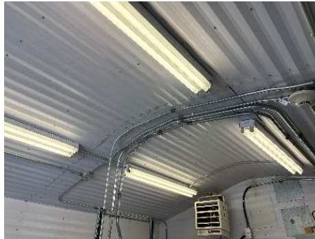
Figure 18: Existing Light Fixture
