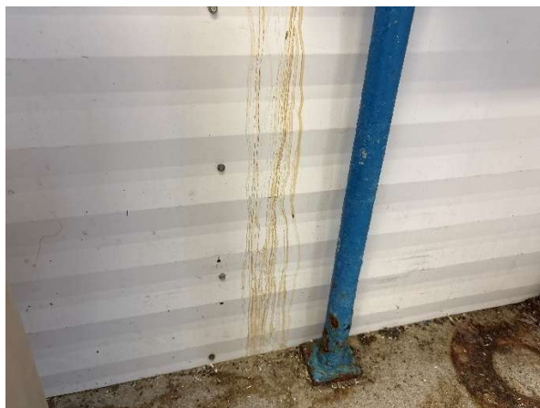
Figure 12: Interior Steel Liner Staining
