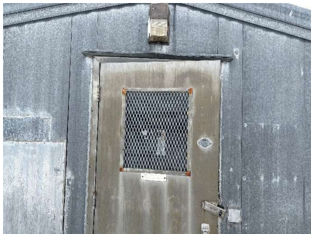
Figure 10: Worn Out Man Door
