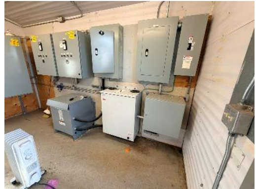
Figure 21: Existing Electrical Equipment
