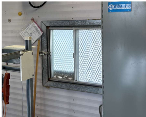
Figure 11: Worn Out Window
