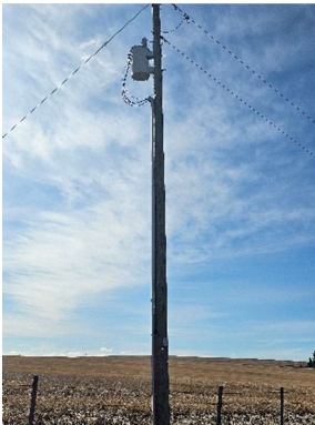
Figure 19: Fortis Utility Transformer
