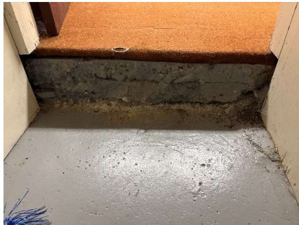
Figure 30: Basement Step Concrete Deterioration
