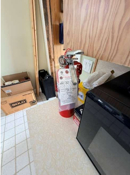
Figure 48: Fire Extinguisher in Kitchenette
