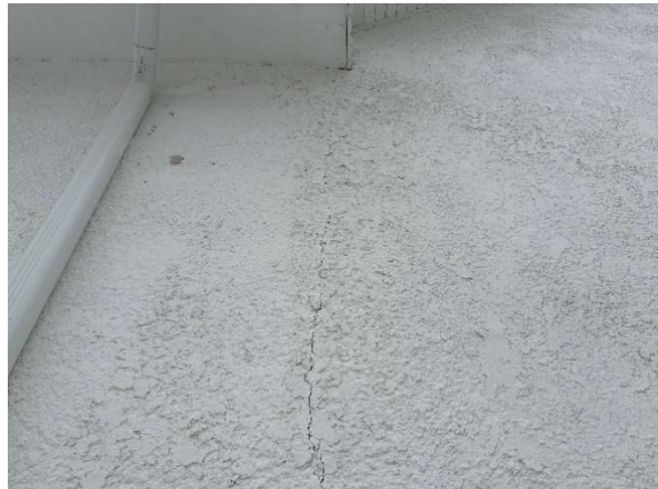
Figure 11: Stucco Cracking at East Stairway Building
