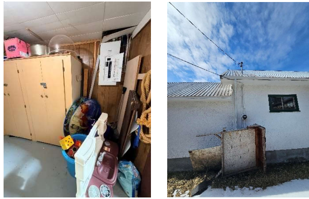
Figure 52: Existing Panel and Utility Meter
