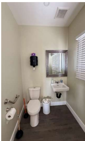
Figure 23: Main Floor Washroom Fixtures
