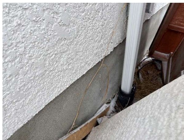
Figure 28: Parging Crack at East Stairway Building Portion
