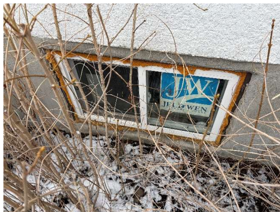
Figure 16: Exposed Spray Foam Insulation Around Window
