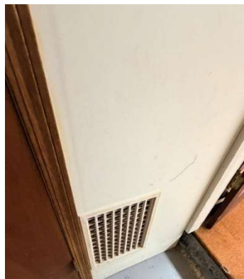
Figure 44: Typical Wall-mounted R/A Grille
