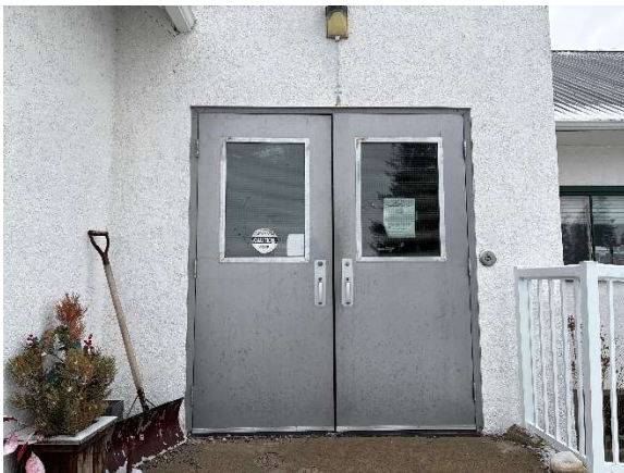
Figure 14: Worn Out Exterior Door
