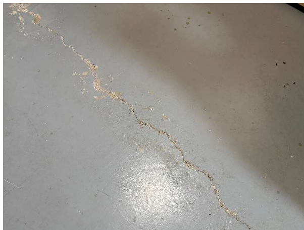
Figure 27: Basement Slab Cracking
