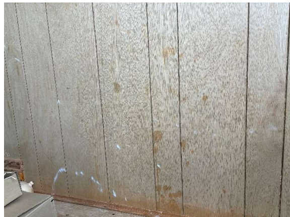
Figure 21: Worn Out Wall Paneling
