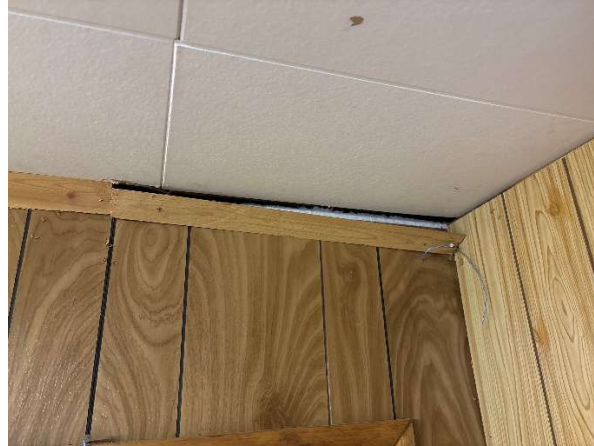
Figure 19: Disconnected Ceiling Trim
