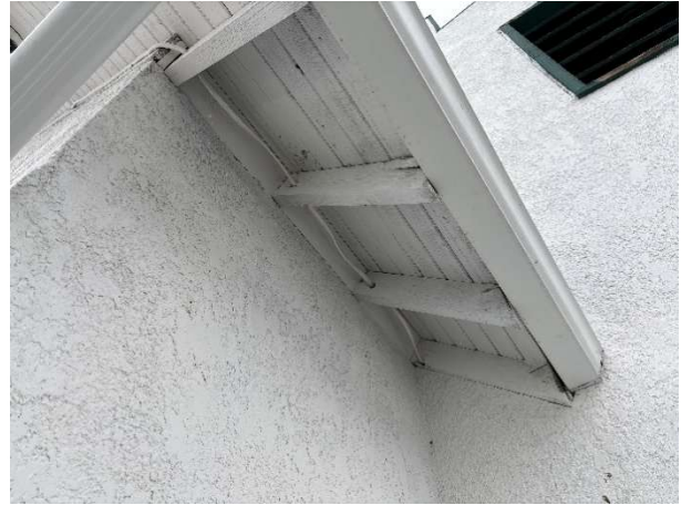
Figure 13: No Soffit Exposing Wires
