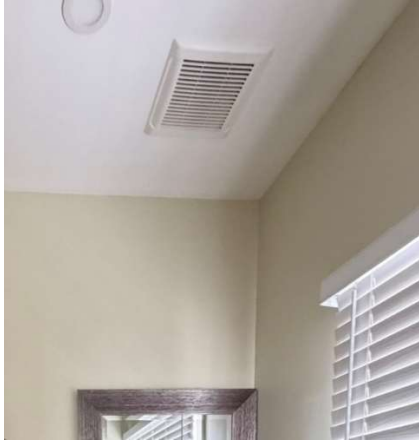
Figure 41: Typical Washroom Exhaust Fan
