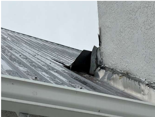
Figure 10: Roof Decking Deficiency
