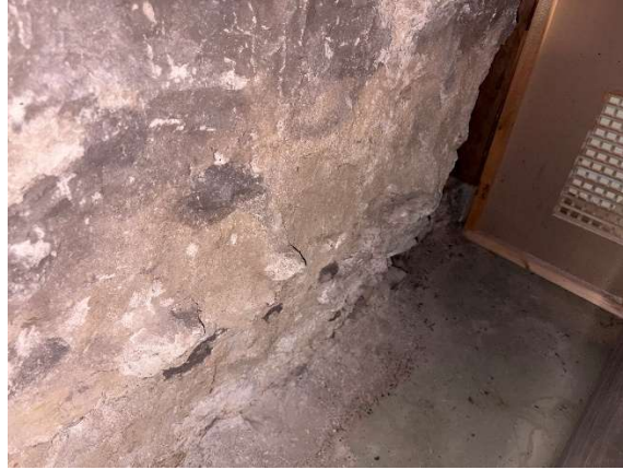
Figure 29: Foundation Wall Crumbling
