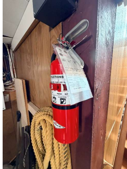
Figure 49: Typical Fire Extinguisher Near Doors
