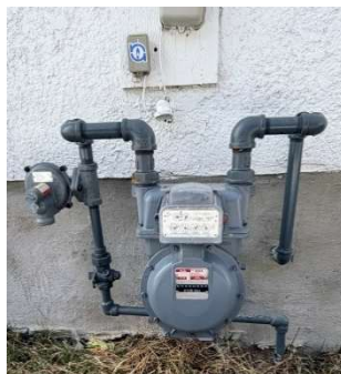
Figure 36: Gas Meter & Regulator SE of Building
