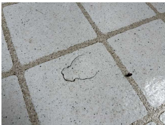
Figure 22: Damaged Laminate Tile Flooring
