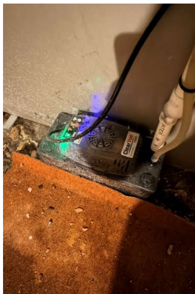
Figure 39: Condensate Pump of Carrier Furnace
