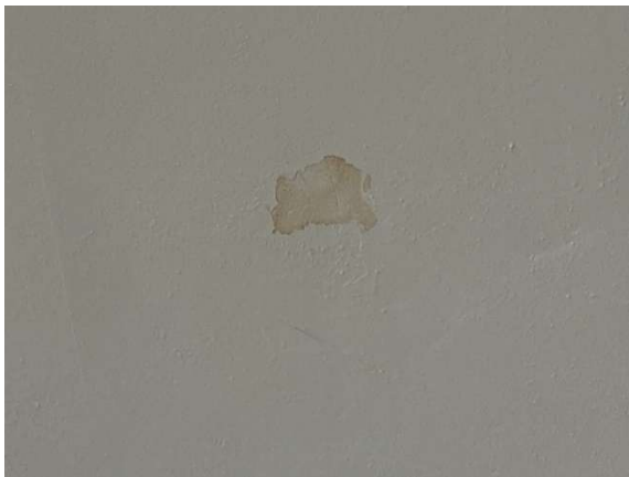
Figure 20: Damaged Wall Drywall
