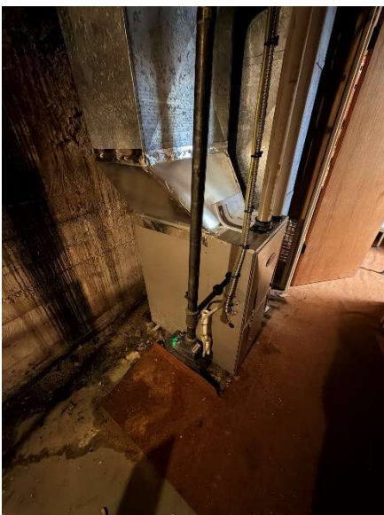
Figure 38: Carrier Furnace in Basement
