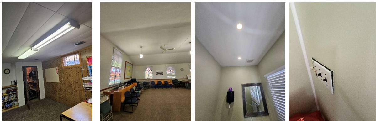
Figure 50: Existing Lighting System
