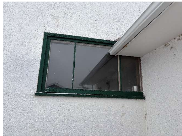
Figure 15: Worn Out Window
