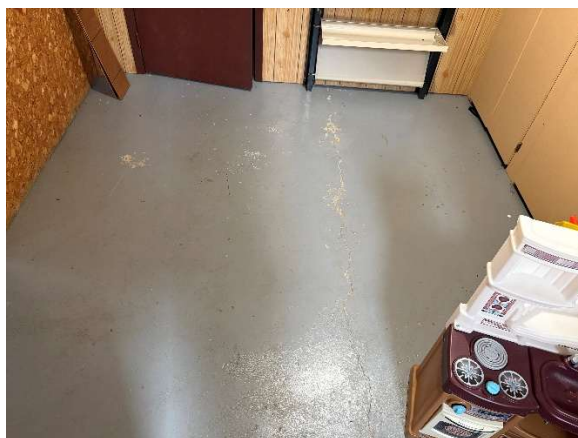
Figure 24: Slab Epoxy Finish Deterioration
