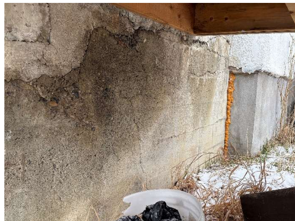
Figure 26: Front Stairway Concrete Deterioration
