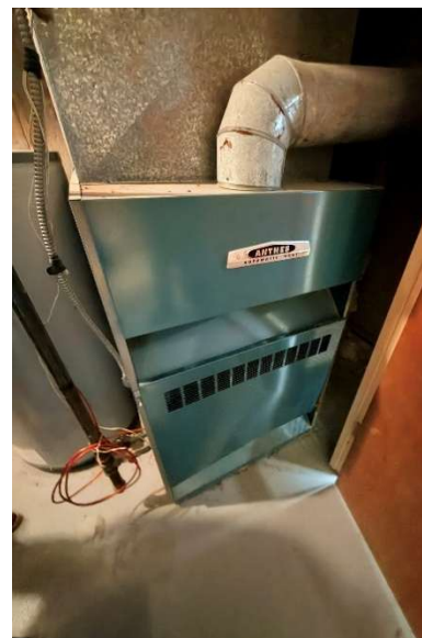
Figure 40: Anthes Furnace in Basement
