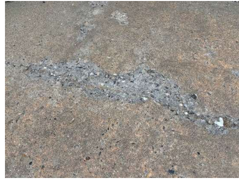
Figure 7: Concrete Stairs Deterioration
