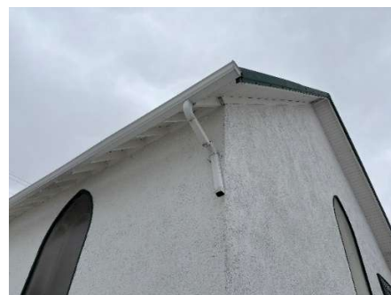
Figure 9: Missing Downspout and Downspout Extensions
