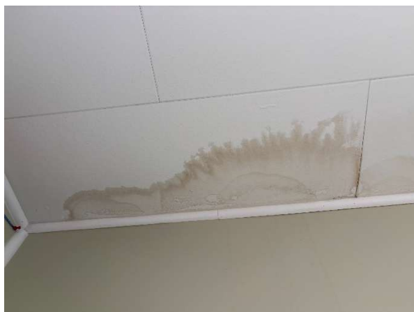
Figure 17: Stained Ceiling Tile
